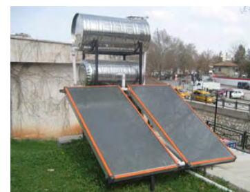
Solar heater on the roof
