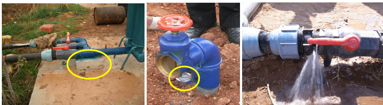
Left: Use of a brick instead of a pedestal makes durability problematic.
