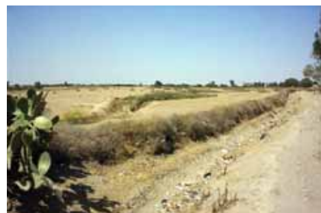
On-farm canal needing repair work
