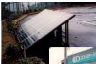
Solar power generator
