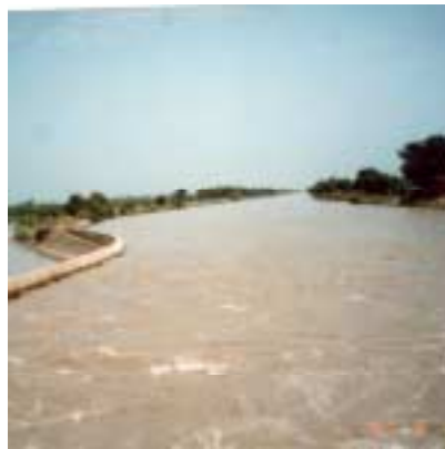
Main irrigation channel
